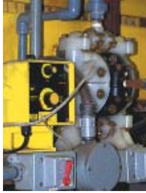
ARO 1/2" diaphragm pumps supply waste water treatment chemicals.
