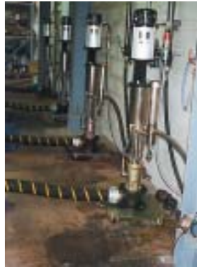
Extrusion pumps used for cold set inks in printing.
