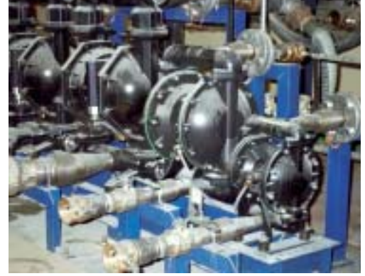
ARO diaphragm pumps transfer bases for paint formulation.
